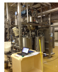
Photo 5. A dosing and mixing tank, discharging into two buffer tanks for feeding two separate production lines.
