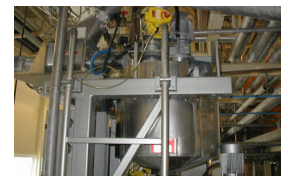
Photo 3. A combined mixing and dosing installation.
