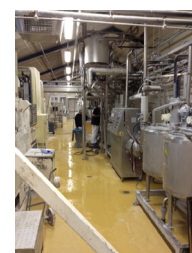
Photo 6. A production line with two buffer tanks and a cooking installation.
