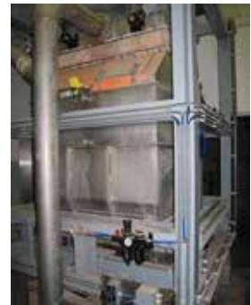
Hopper weighing system
