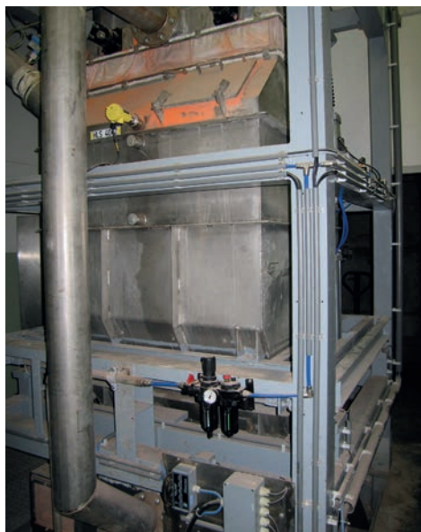
Fig. 1 A hopper weigher for fertilizers, with a capacity of 3,000 kg and an accuracy of 3,000 d or 0.03% (a read out per 1 kg). The installation can reliably dose quantities from 20 kg off
