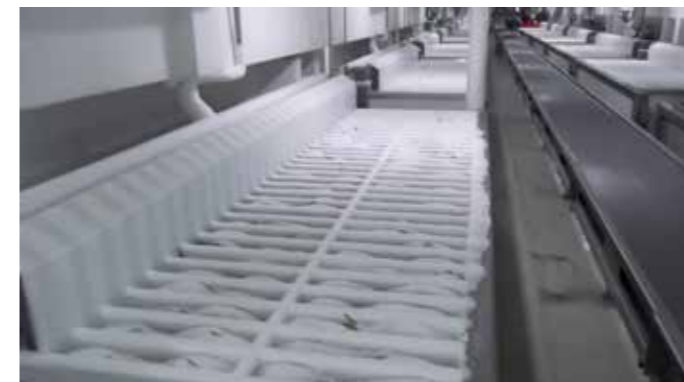
The frosters previously were overfilled
