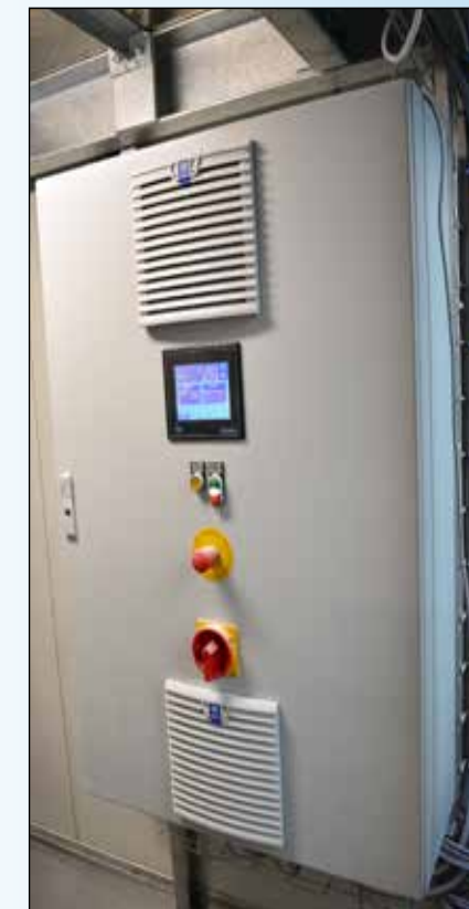
The batch controller to which the two trays (scales) are linked
