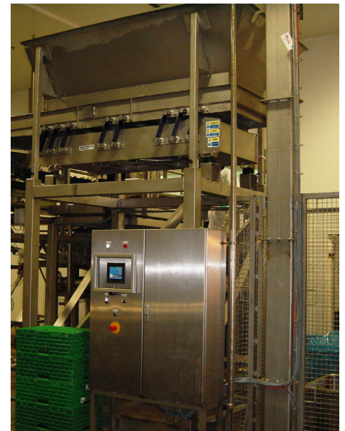
in spite of the relatively high mass of the belt conveyor a system with a weight controller could be realized.
