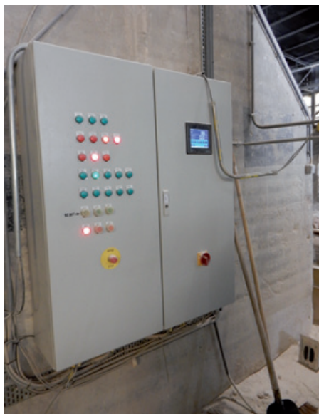
Fig. 4 The control panel with the weighing controller
