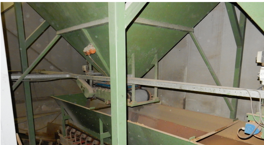
Production facility with counterflow mixer and cement weigher
