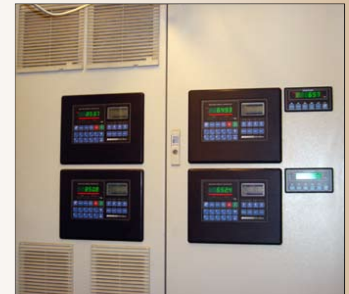
the control panel
